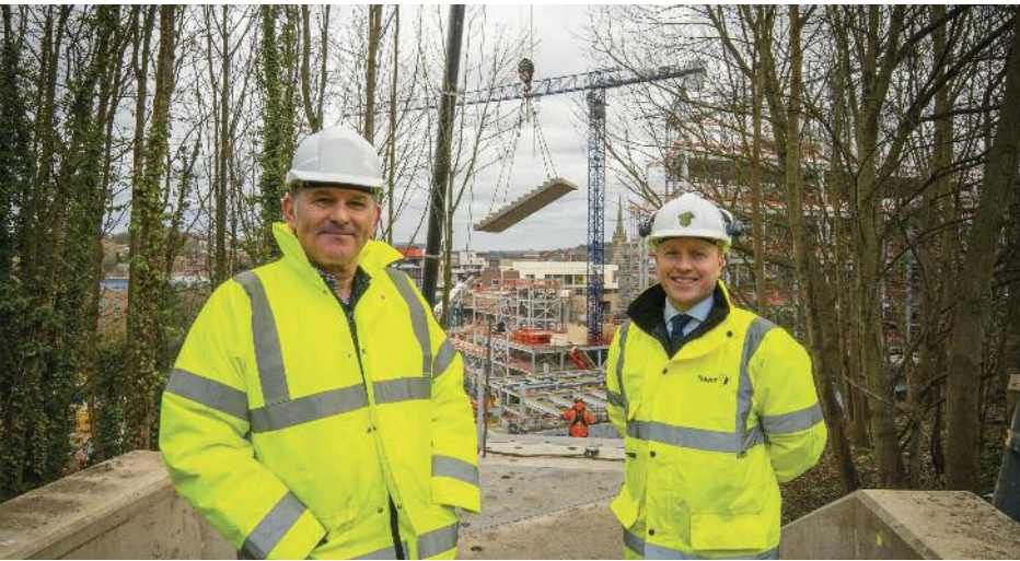
Allan Cook and Paul Salked at the top of the new staircase as one of the sets of concrete steps are lowered into place.
